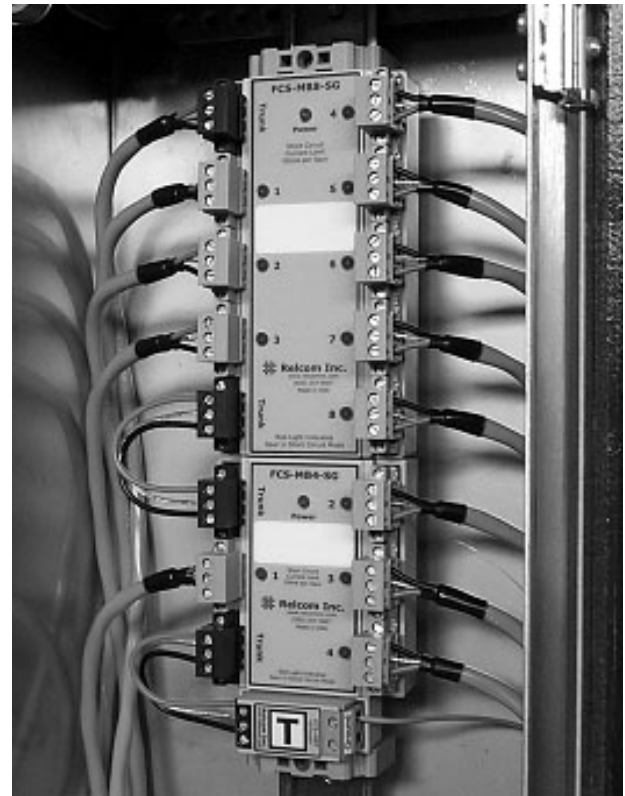
Fieldbus Junction box wired for 12 devices including a Terminator
